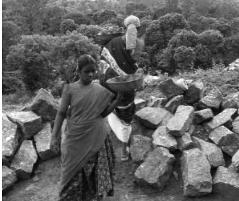
An Irula women's group in southern India building their new Village Resource Centre, initiated by Keystone. Here they will be able to improve their income through value-addition from non timber forest products.
